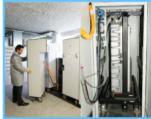
B4B project - Batteries for buildings Storing energy in buildings
